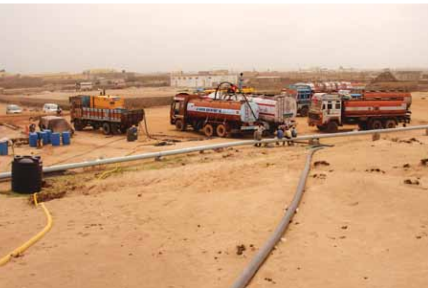
Offloading fuel oil from vessel through makeshift floating pipeline and on to trucks.
